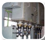
Power sensitive equipment
