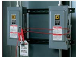
Lockout single or multiple electrical disconnects
