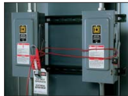
Lockout single or multiple electrical disconnects
