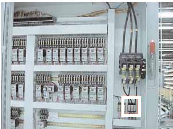
PDB in UL 508A, 480V Feeder Circuit must have spacing of 1” through air and 2” over surface. PDBs listed to UL 1953 meet these spacing requirements. Terminal Blocks recognized to UL 1059 must be verified to have required spacing.
