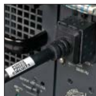
Electrical Infrastructure Labeling
