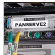
Network Infrastructure Labeling
