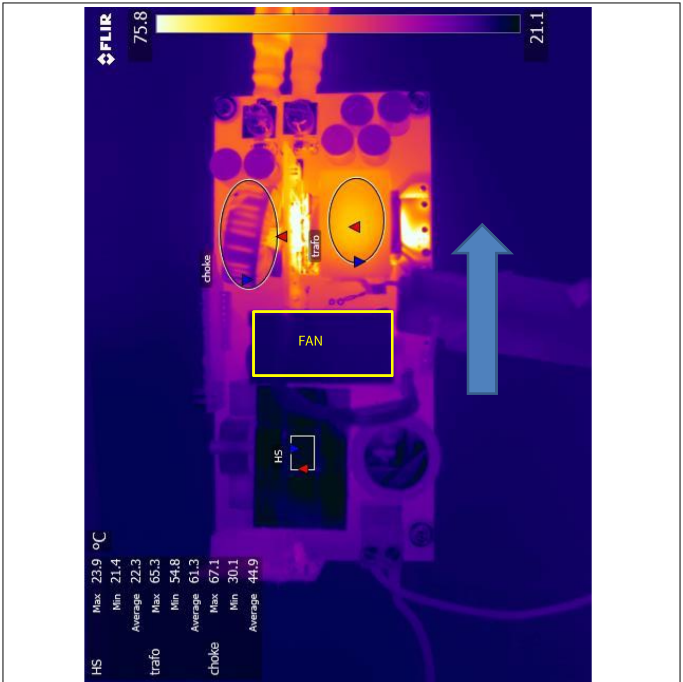
Figure 80 Board thermal map at 100 percent load (117 A) at room temperature (~24°C)
