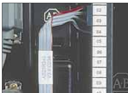
Terminal Block Labeling
