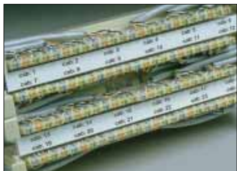
Network Systems Labeling
