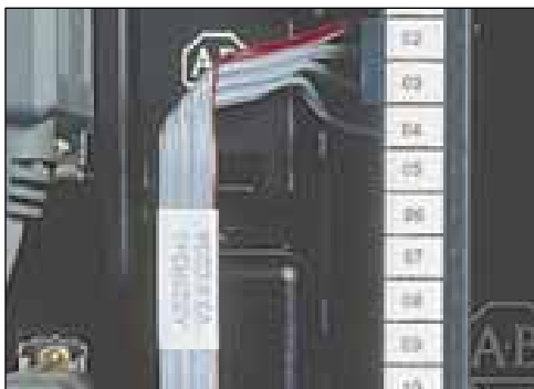
Terminal Block Labeling
